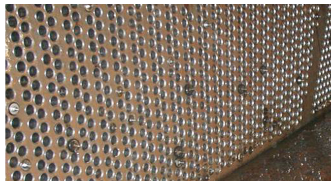
Tube condition with debris filter
