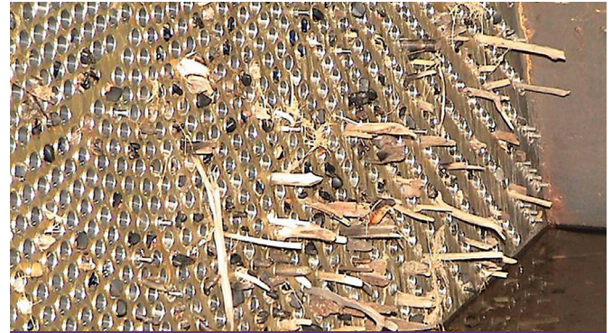
Condenser tubes without debris filter
